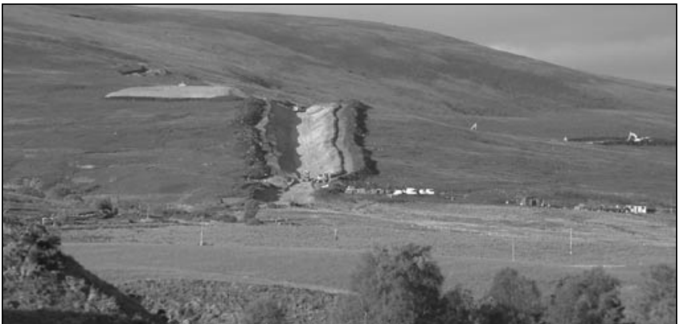
Access roads to Paul's Hill Wind Farm are under construction ( Bob Laughton )
