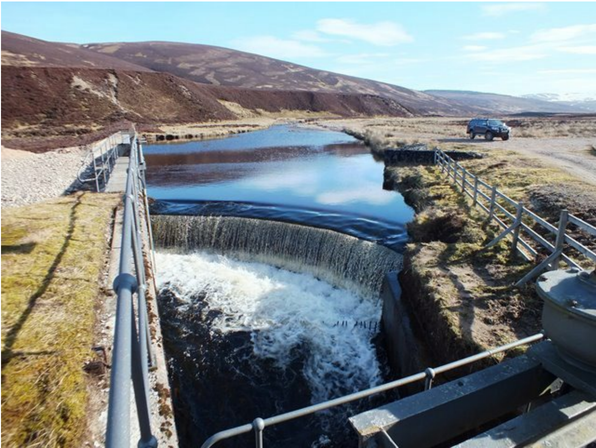
Above: The water off-take at the Allt Bhran, the most significant tributary of the River Tromie. All of the Allt Bhran's flow is diverted into the Tromie Dam, most of which is then sent on in to the Tay catchment to generate hydro-electricity. (Photo: Brian Shaw)
