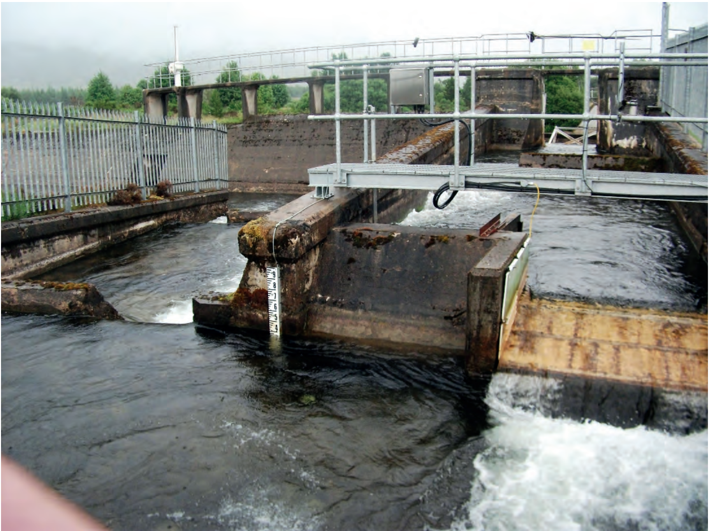
Above: Scottish & Southern Energy's water off-take and fish pass (with resistivity counter) on the River Truim, near Dalwhinnie. It is from here that water from the River Truim is diverted into Loch Ericht and then in to the Tay catchment, for the production of hydro-electricity. (Photo: Roger Knight).
