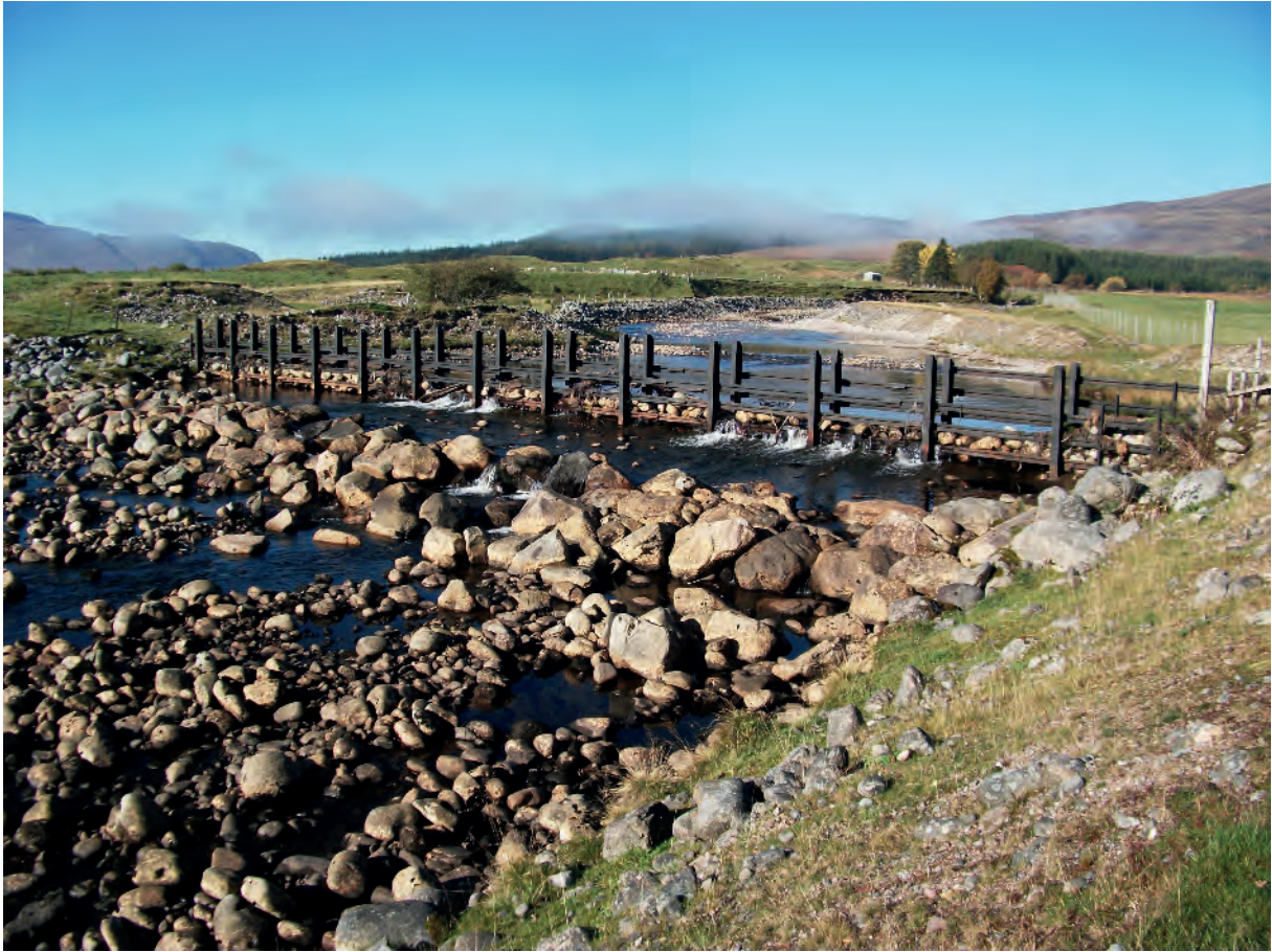
Above and below: The heck across the River Markie, a tributary that joins the River Spey immediately above Spey Dam. The heck is designed to prevent gravel transported by the River from accumulating behind the Dam. However, it also prevents spawning fish from accessing the River Markie. (Photos: Roger Knight).
