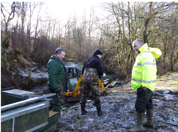
Construction Team at work: Alistair Grant, Josh Walker, Jason Hysert and Lindsay Grant. (Photo Courtesy of Richard Whyte)
